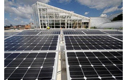
125kW Solar Array at Phipps Conservatory
